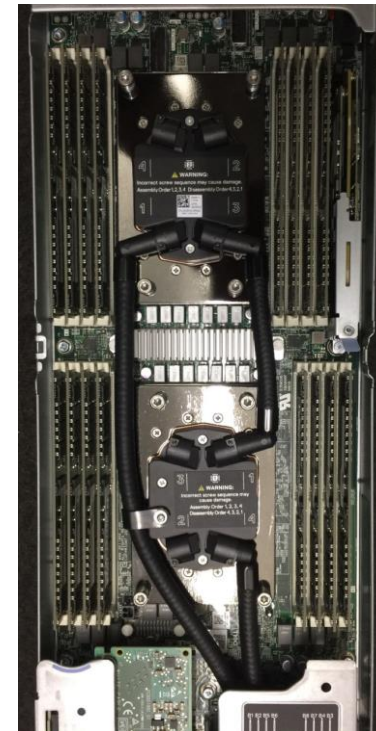
Interior of CPU worker node
