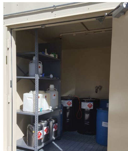
To safely expand the NSRL's ability to store the bulk quantities of ethanol required to curate the collections, a new chemical storage facility for the NSRL has been constructed.
