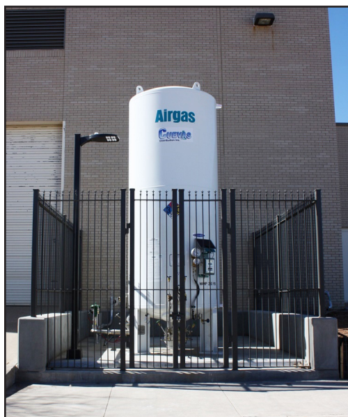
The 1,500-gallon bulk tank installed outside the NSRL building automatically supplies the freezers with liquid nitrogen via a vacuum-jacketed piping system.
