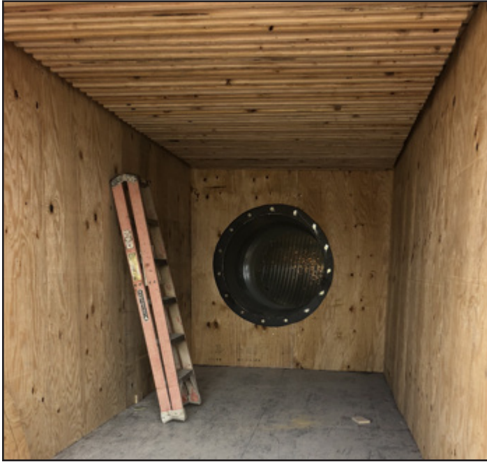
A view inside the artificial cave under construction, showing the slatted roof that will provide roosting sites.
