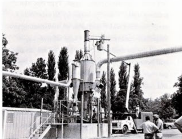
FIGURE 6. Heat-recovery incineration system during stack emission tests.
