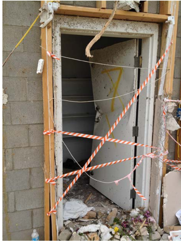
Mayflower, Arkansas Door Damage
