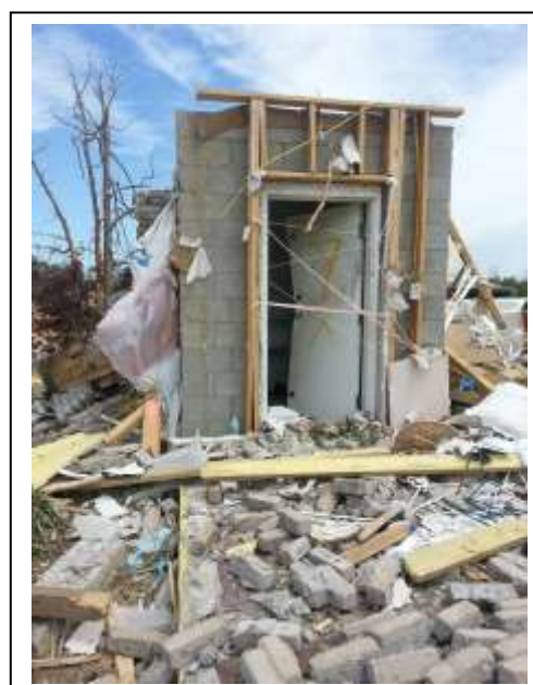
Surviving above ground shelter with failed door
