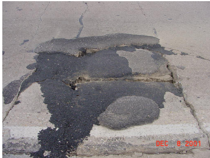
Figure 7. Punchout distress with tight crack width
