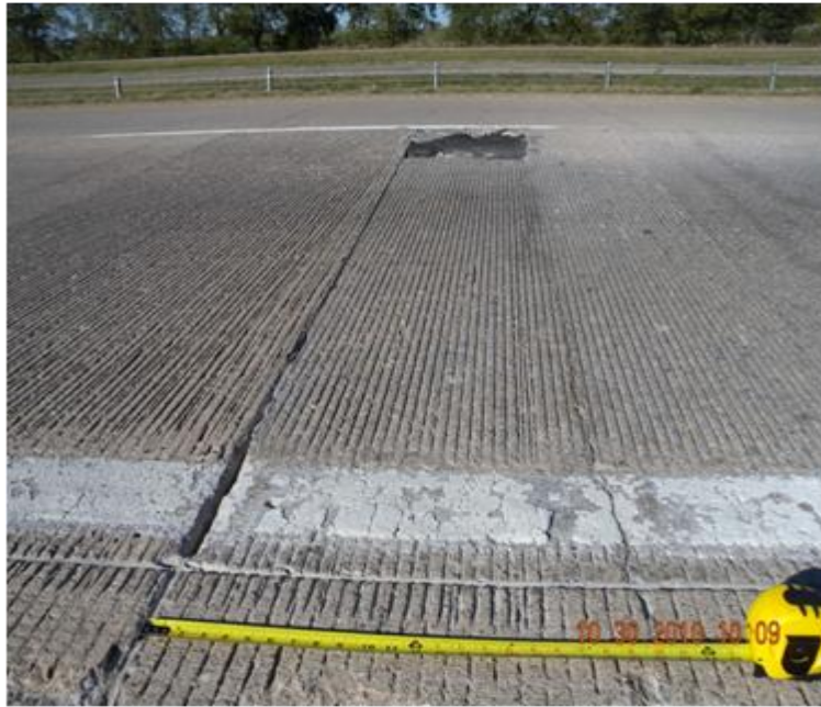
Figure 10. Distress at transverse construction joint
