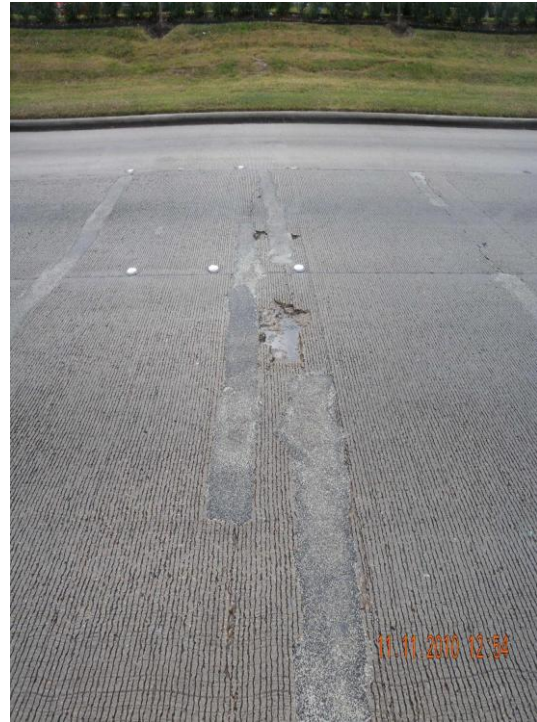
Figure 2-(b) Spalling and repairs
