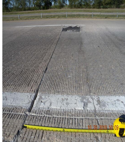
Figure 4-(b) Distress at transverse construction joint
