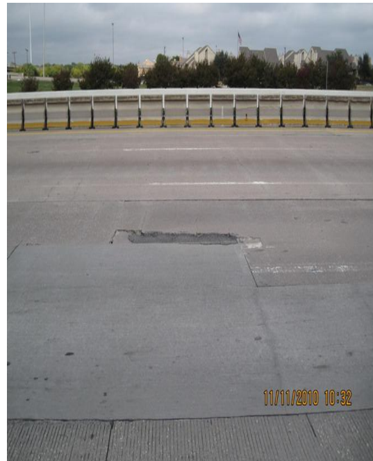
Figure 3-(b) Distress at repair joint
