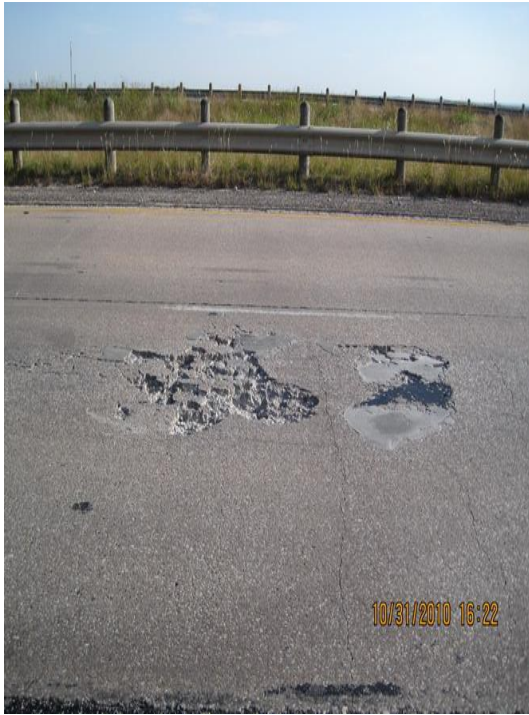
Figure 2-(a) Large surface defect
