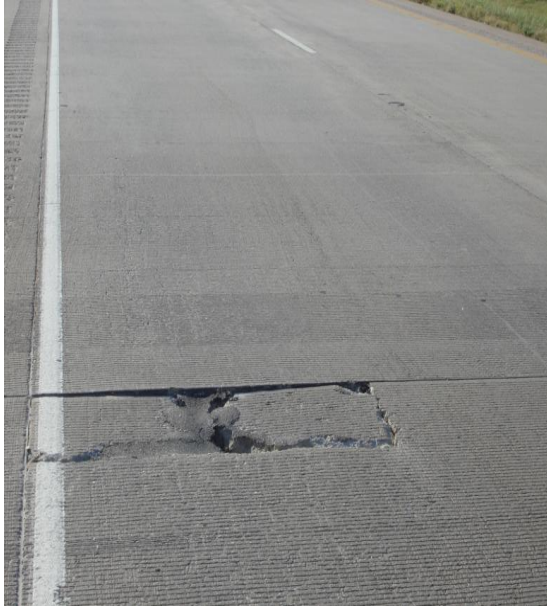
Figure 4-(a) Distress at transverse construction joint
