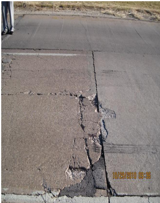
Figure 3-(a) Distress at repair joint
