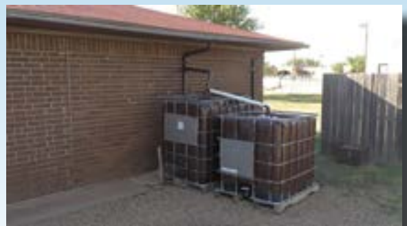
Storage for the water harvest system.
