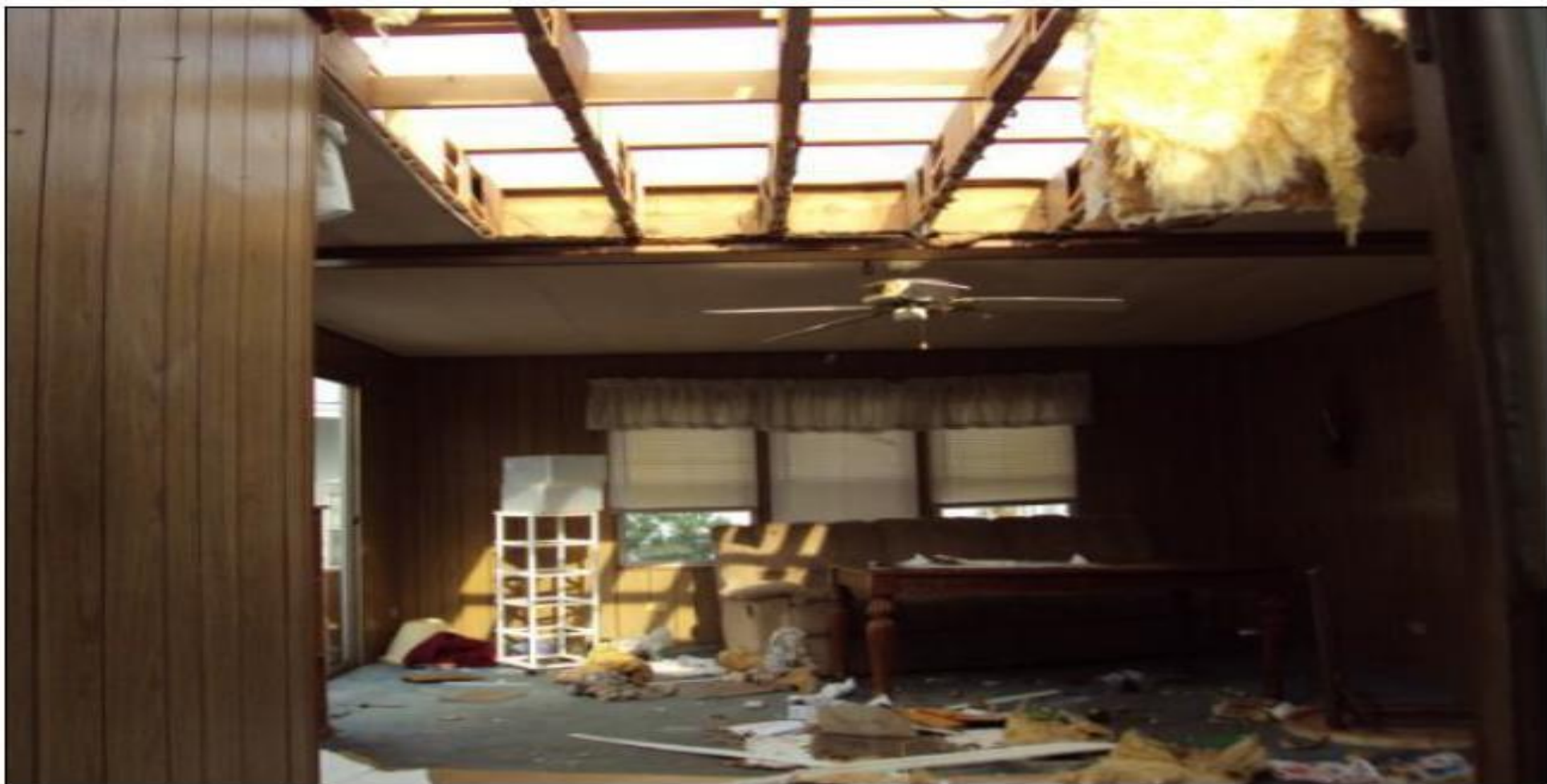
Interior damage typical of FEMA-assessed DS2+ homes.
