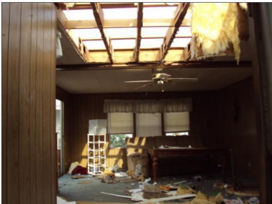
Example of interior damage of DS2+ severity
