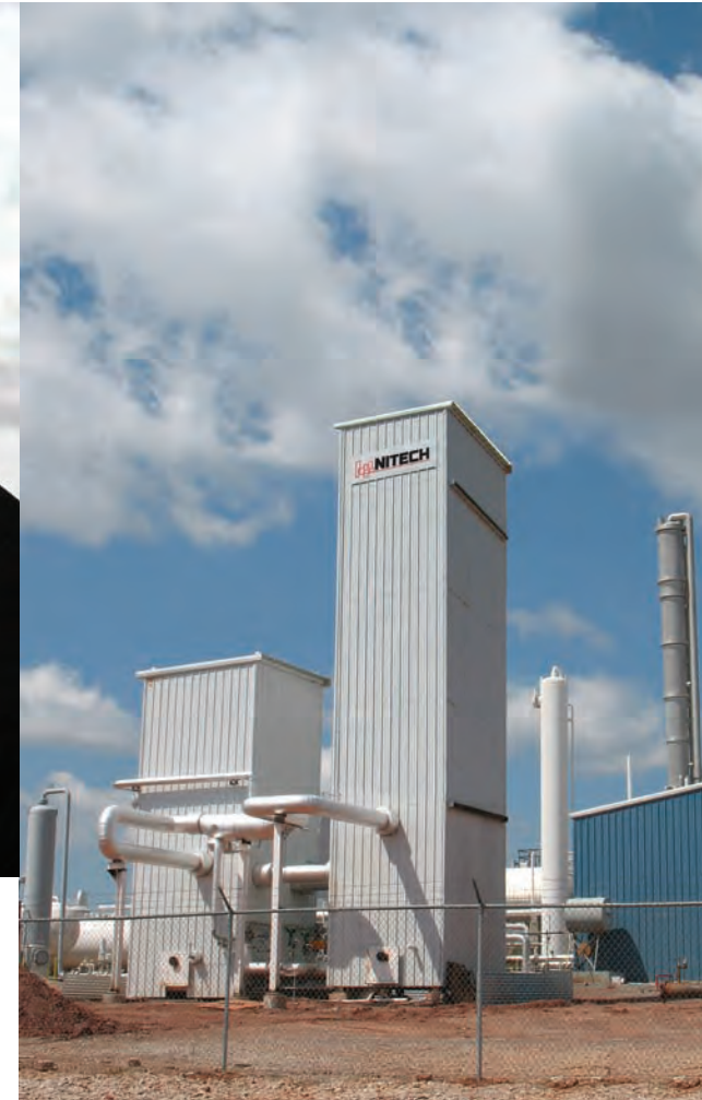
(Above and right) BCCK facilities for nitrogen rejection, NGL recovery, CO 2 removal, helium recovery, and oxygen removal.
