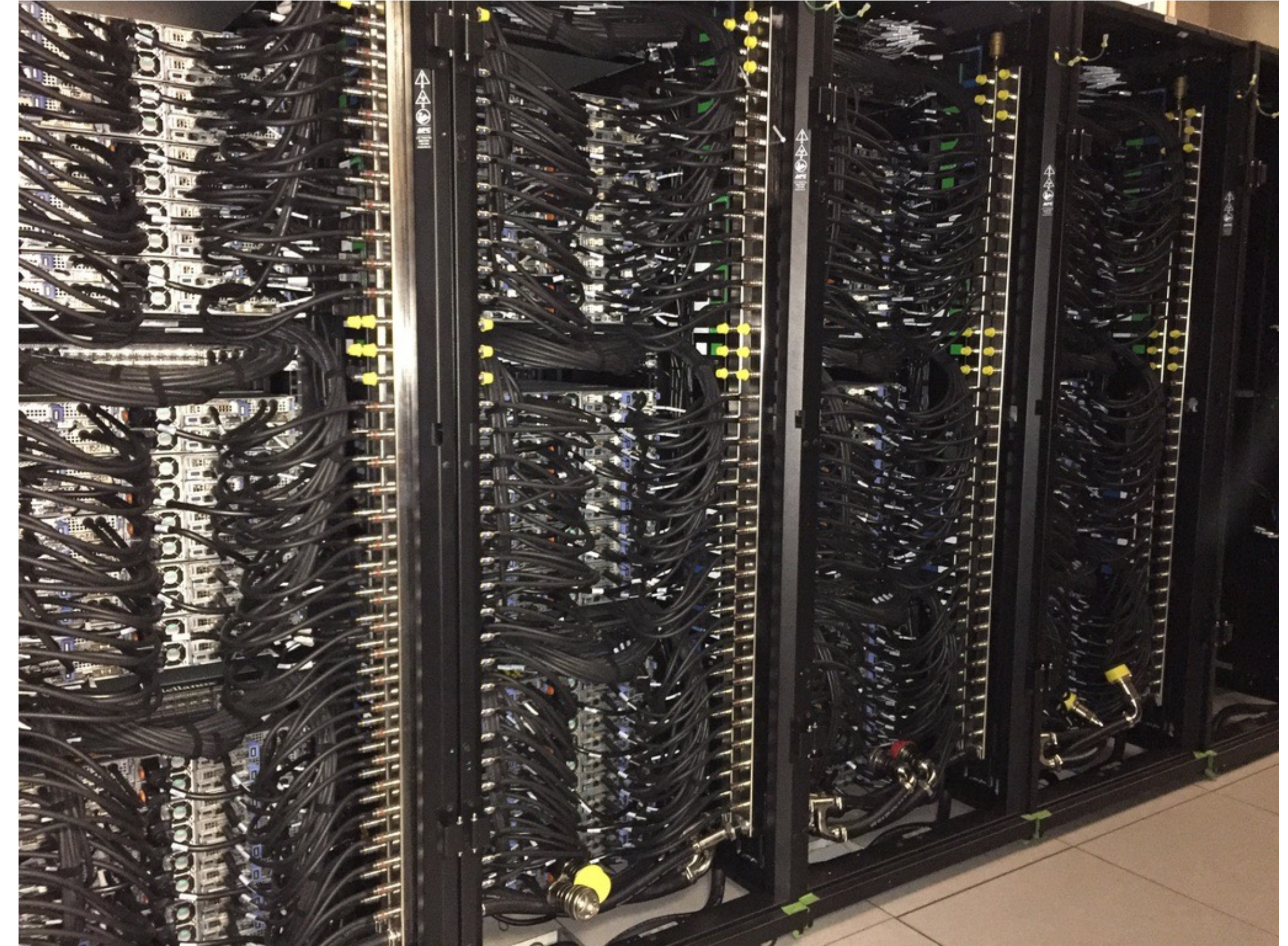
Back view - CPU racks
