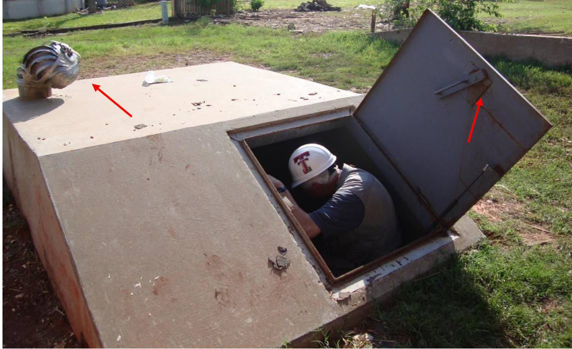
Figure 1.8. Clam shell shelter with an insufficient locking system and damaged vent at an EF-2 rated location (No. 3).
