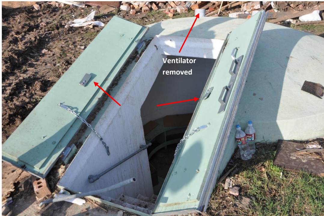
Figure 1.14. Dome shelter with an inadequate door system that included a plywood and lite gauge sheet metal clad door, single locking point, and ventilator removed at an EF-3 rated location (No. 43).
