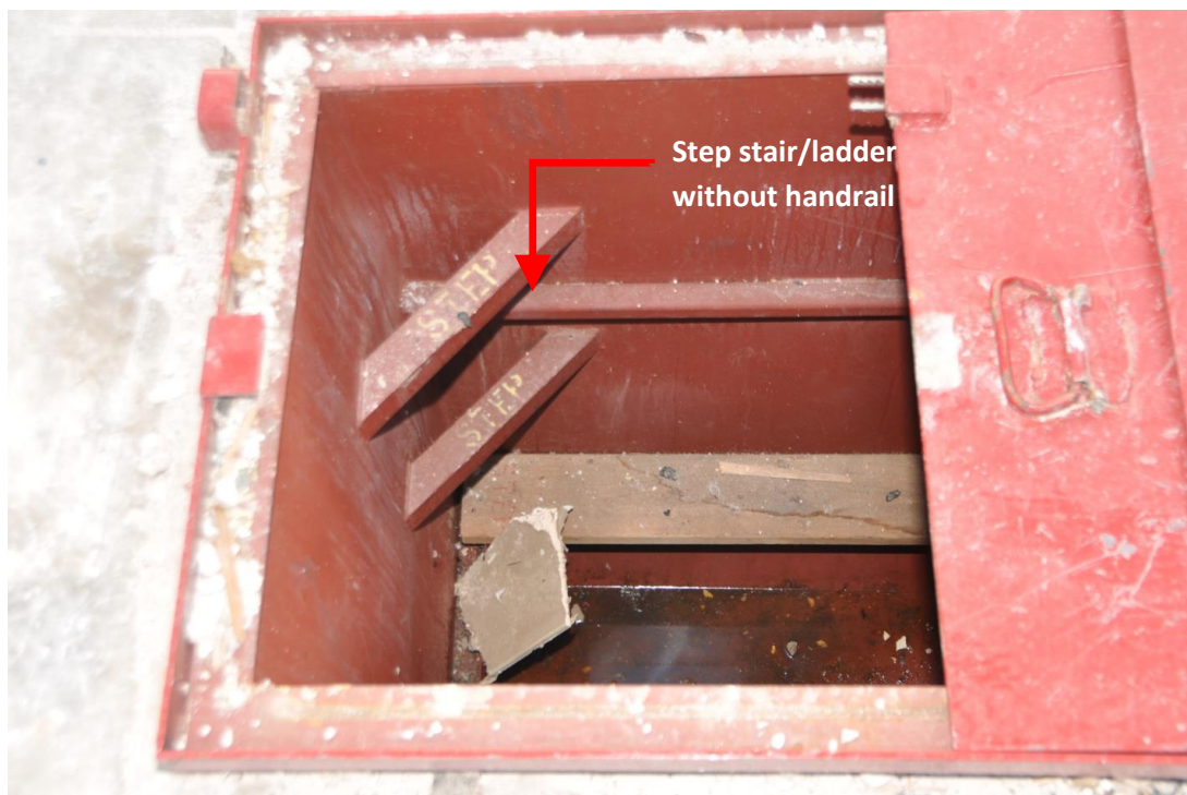
Figure 1.11. In-garage storm shelter with inadequate stairs, locking system, and flooding in the bottom at an EF-3 rated location (No. 12).
