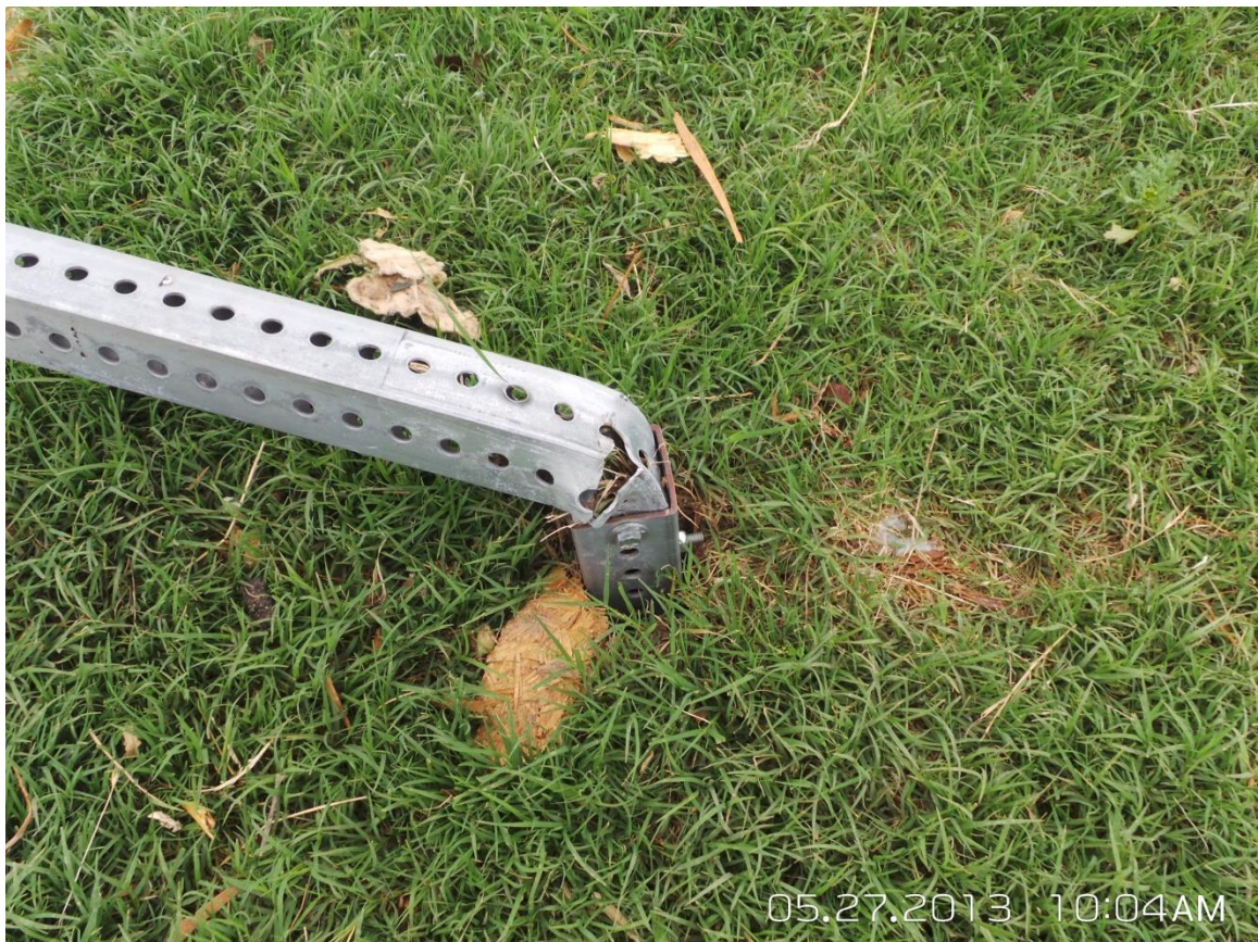
Figure 2.9 Bending failure of post for structure 2, stop sign.
