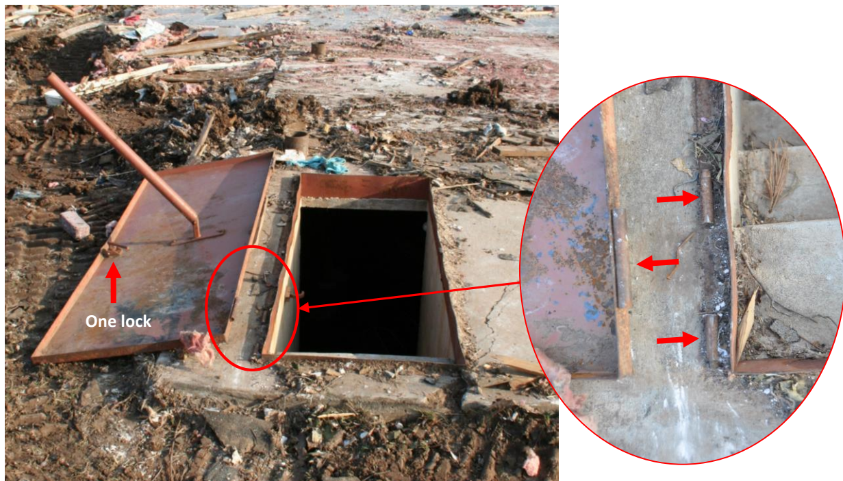
Figure 1.7. Door failure of shelter with only a single lock point (No. 47).
