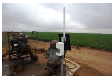
Surface turbine irrigation well
