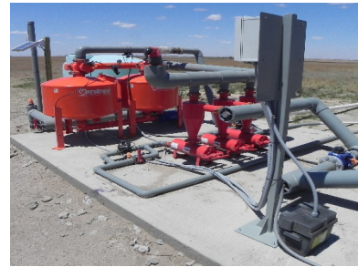
SDI filtration system
