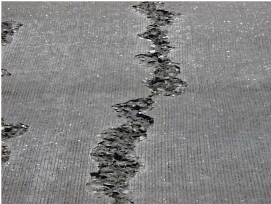
FIGURE 7 Spalling in CRCP with virgin siliceous river gravel.
