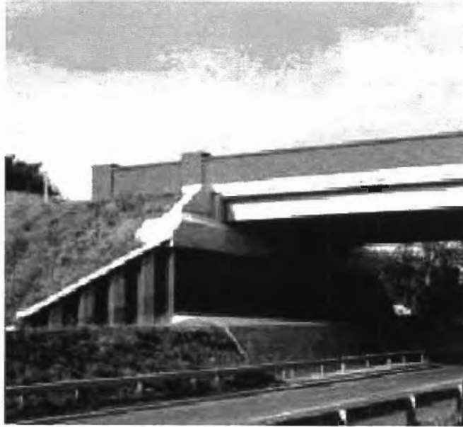
Figure 5.12 Use of Permanent Steel Sheet Pile Walls for a Bridge Abutment (Source: Steel Construction Institute, UK)
