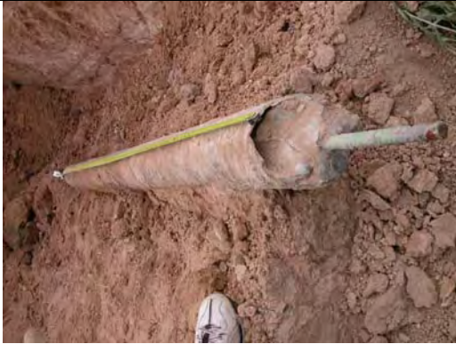
Exposed Nail #5 Bad head condition, only 1/2 of nail head is grouted
