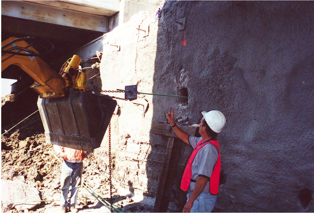
Figure 2.16 Low Pullout Strength Due to Incomplete Grouting
