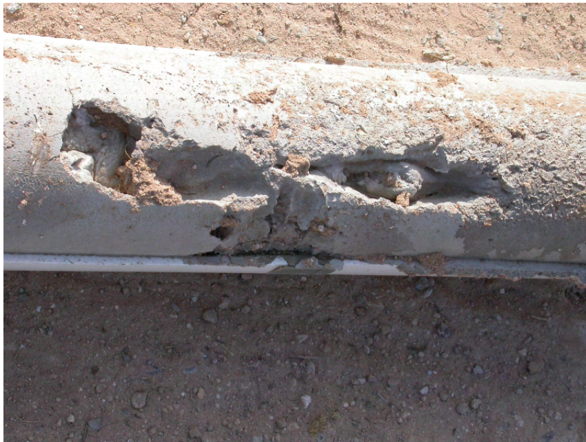
Figure 6.14 Sand Grout Column with a Defect Caused as an air Pocket was Formed during Grouting
