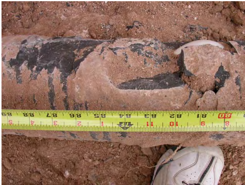
Figure 5.49 A minor defect on Nail 5 at 7 ft
