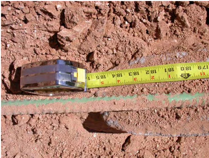
Figure 5.37 Nail 29 - Grout Stops at 15.3ft
