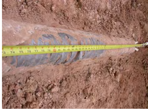
Grout goes through the middle defect, ends at 11'4"
