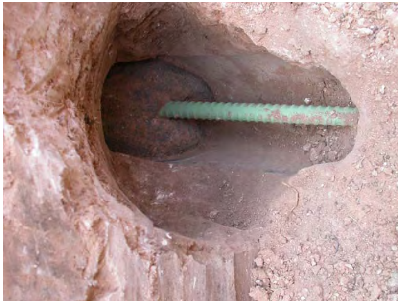
Figure 4.29 Incomplete Grouting of Test Nail No. 23
