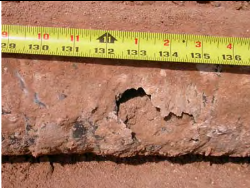
Minor defect at 11'1"
