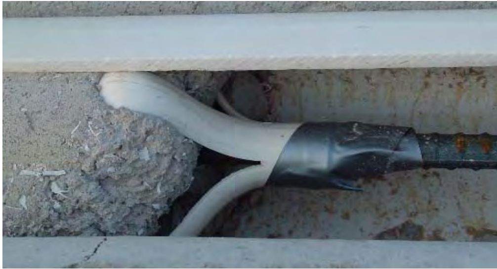
Figure 6.11 Sand 1 Grout in Tube 8, Showing Middle Centralizer and Distant End of Grout Column
