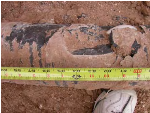
Minor Defect (area reduction) at 7'
