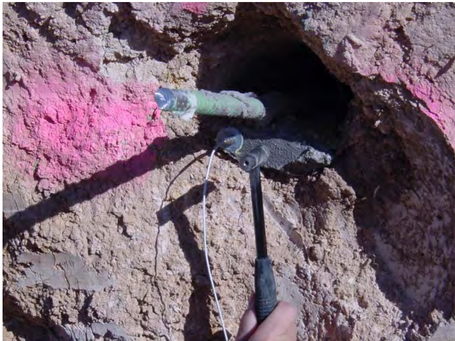
Figure 5.7 Sonic Echo and Impact Echo Test Configuration: Accelerometer Mounted on the Grout, Impact on the Grout with the Alumina Tip
