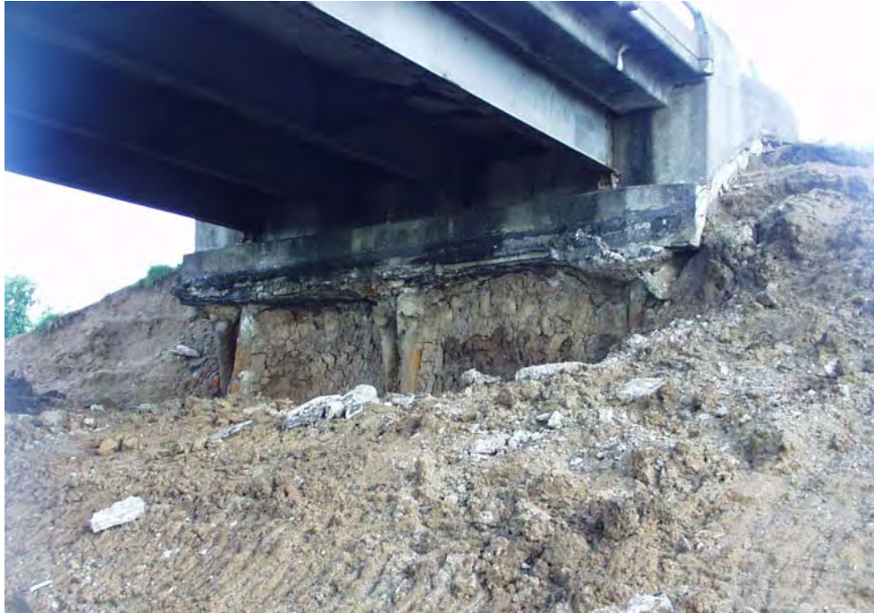
Figure 2.8 Face Sloughing Caused by Unnailed Cut Left Exposed for a Long Period of Time
