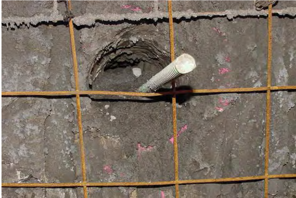
Figure 2.20 Bird Mouth Defect Caused by Poor Grouting
