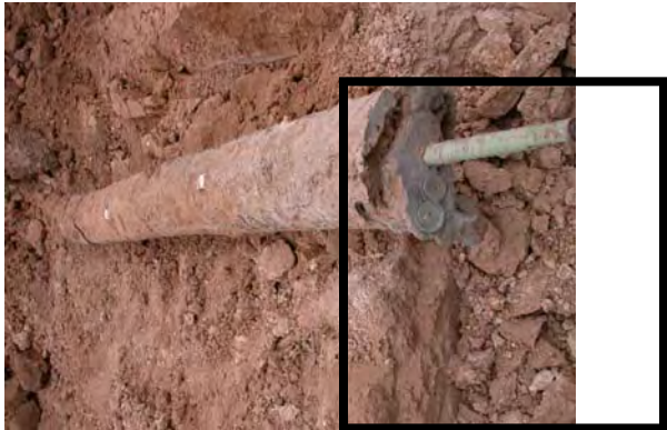
Exposed Nail #15 Nail ends at 5.5 feet, bad head condition
