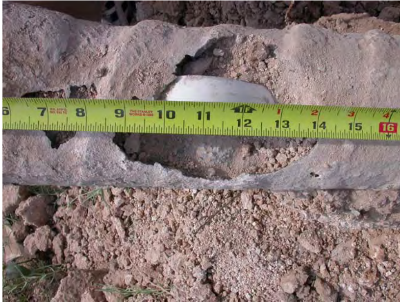
Figure 5.45 Shallow Defects Found in Nail No.16
