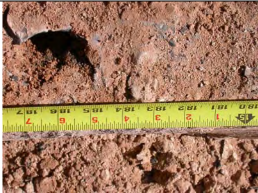
Minor defect at 15'5"
