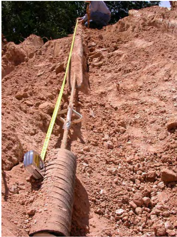
Figure 5.36 Exposed Nail #29 (Grout Did Not Reach Foam Obstruction)
