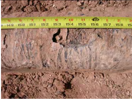
Minor defect at 12'10"
