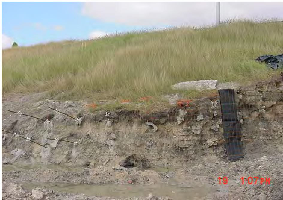
Figure 2.9 Face Instability Caused by Unnailed Cuts Left Exposed for a Long Period of Time
