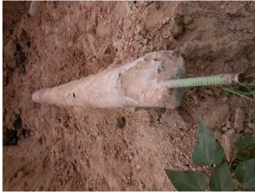
Exposed Nail #4 Bad head condition, only 2/3 of nail head is grouted
