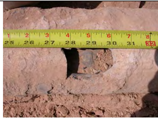
Minor defect at 2'5"
