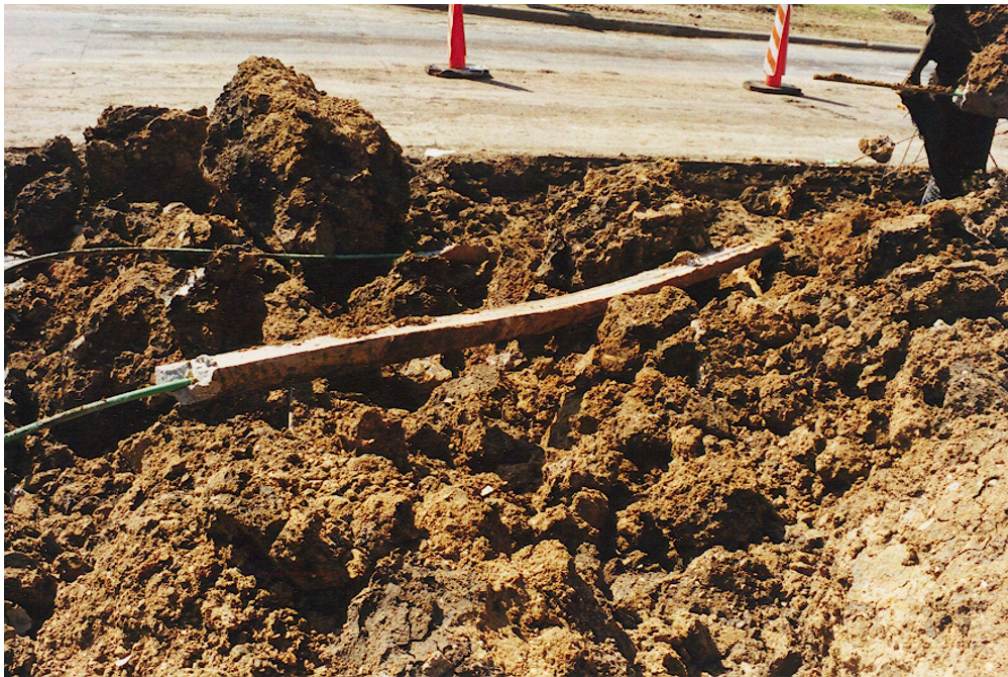
Figure 2.15 Pullout Caused by Drillholes Half Filled with Grout
