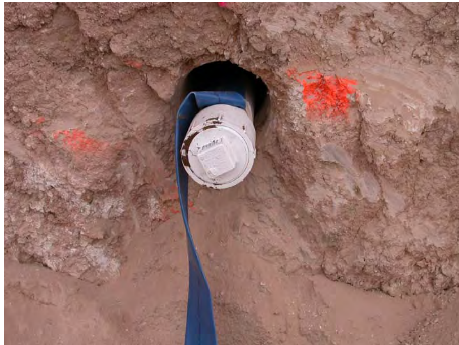
Figure 4.25 Flexible Hose Used for Placing Bentonite Grout Around PVC Access Tubes (Parallel & Cross-Hole Seismic Tests)
