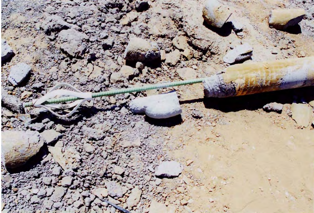
Figure 2.22 Void at the End Caused by Incomplete Grouting
