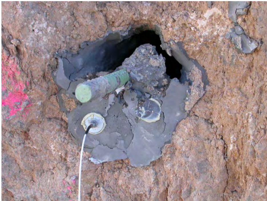
Figure 4.28 Nail Head in Poor Condition
