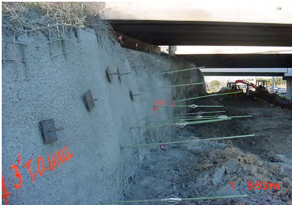
Figure 2.21 Insufficient Tendon Length Caused by Nail Hole Caving
