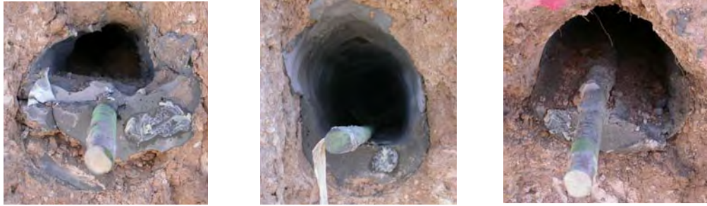
Figure 5.46 Bird's Mouth Defects in Nails 2, 20 and 4 that Limit the Proper Access
