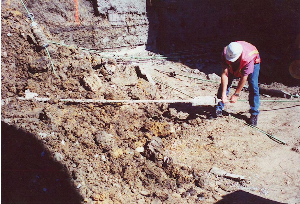
Figure 2.14 Pullout Caused by Incomplete Grouting
