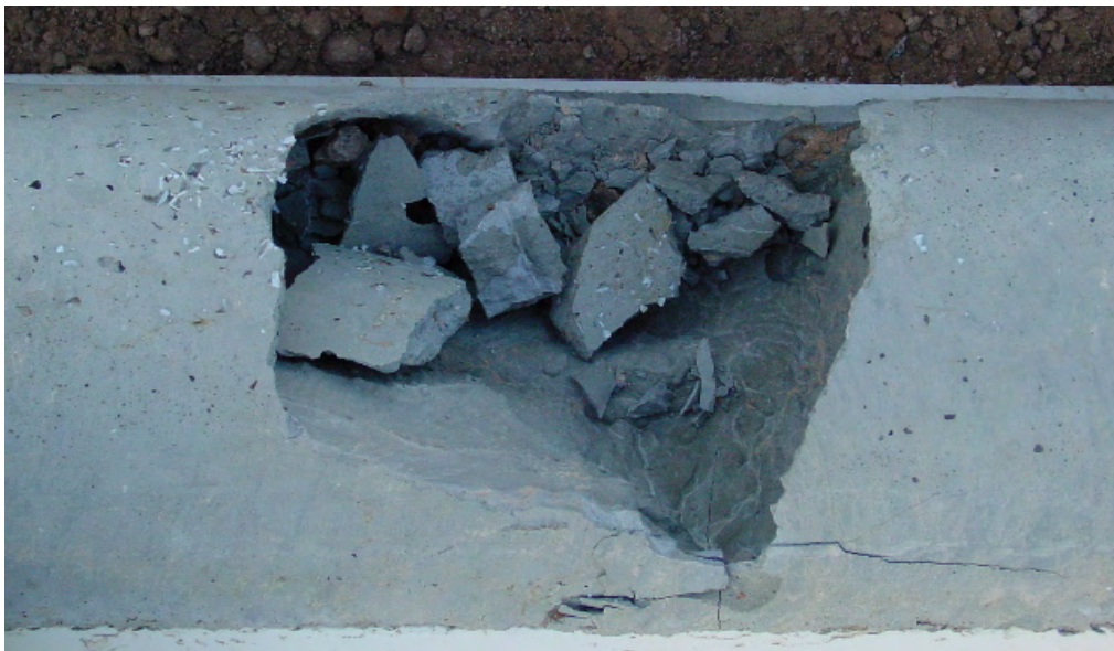
Figure 6.12 Neat Cement Grout In Tube 1, Showing A Void Across About \frac{1}{2} Of The Grout Column Diameter
