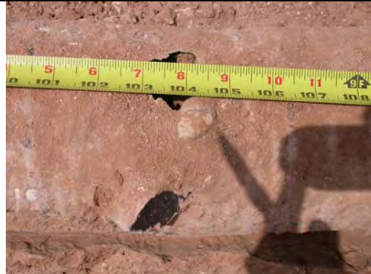
Minor defect at 8'8"
