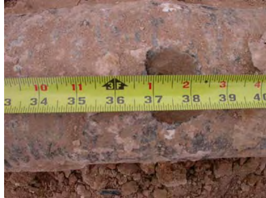
Minor defect at 3 ft
