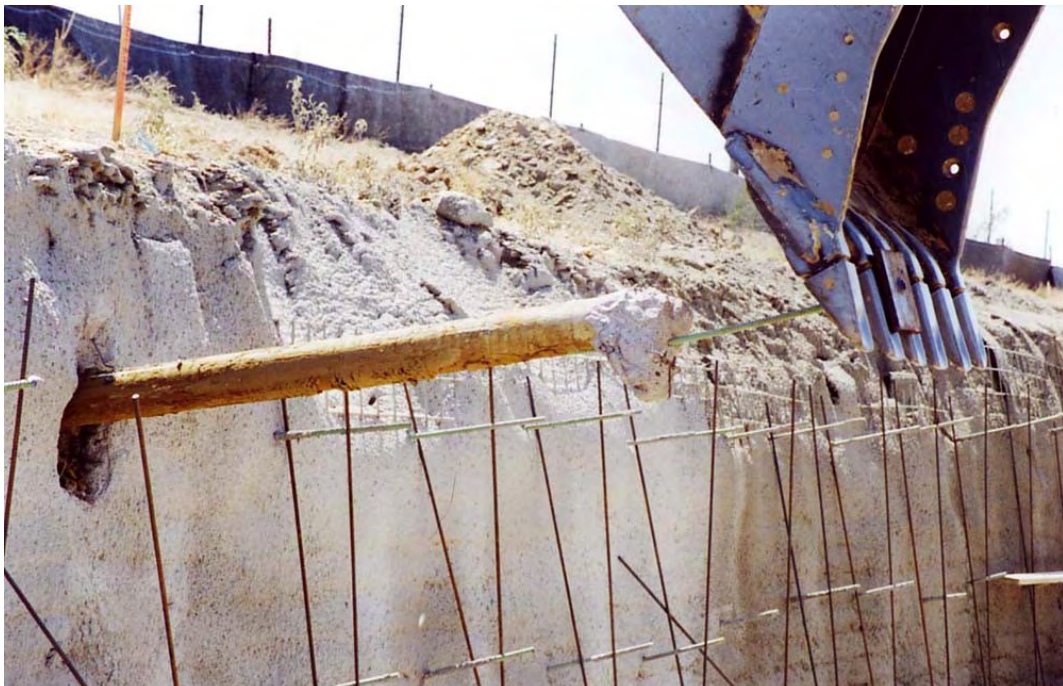
Figure 2.17 Off-Center Tendon Due to the Use of Too Few Centralizers
