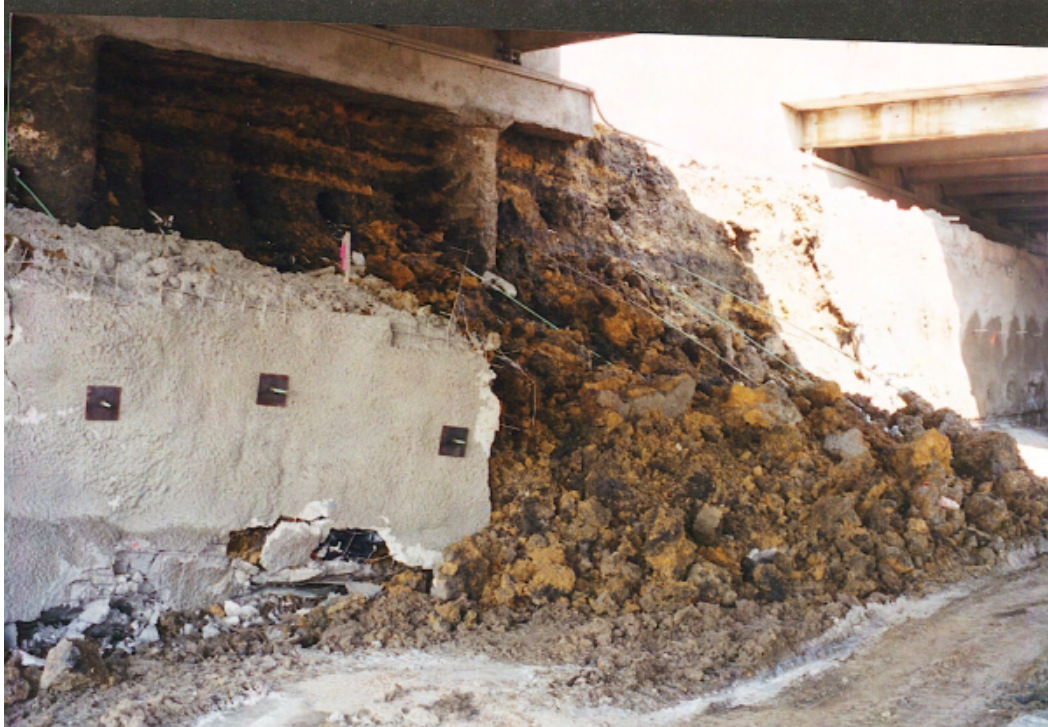
Figure 2.12 Failure of Wall Caused by Incomplete Grouting
