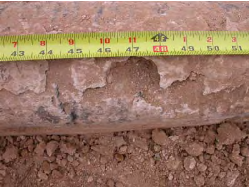
Minor defect around 4 ft
