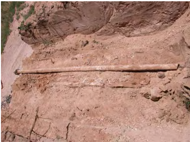
Figure 5.31 Exhumed Nail No.26
