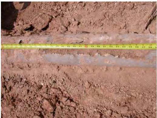
Minor defect around 3'3"-4'8" area
