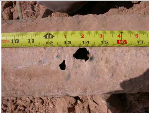
Minor defect at 1'2"
