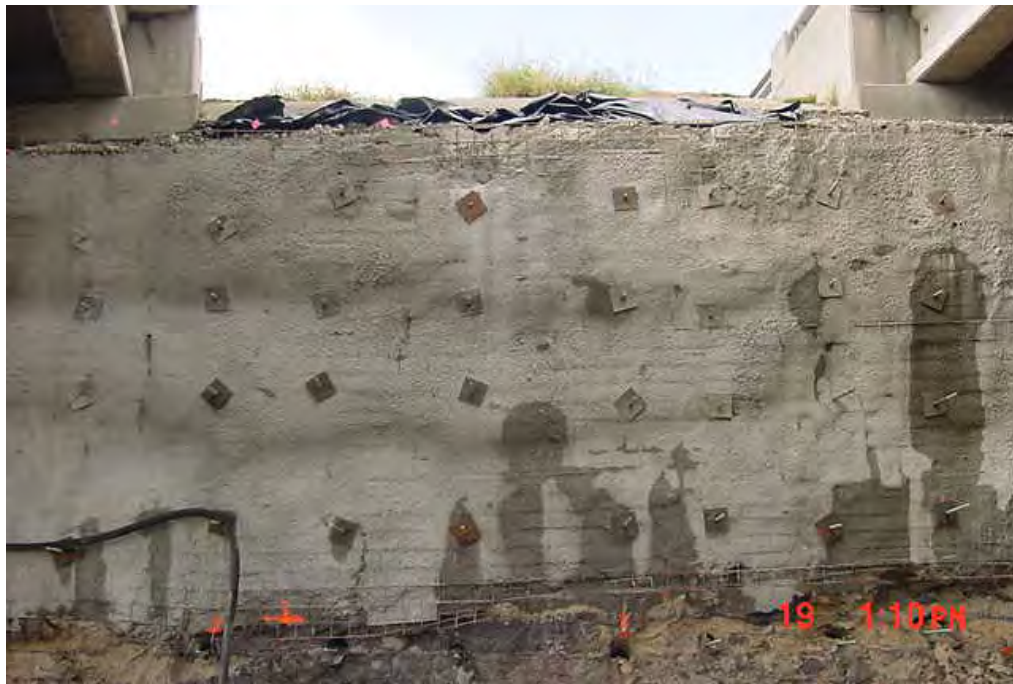
Figure 2.11 Washout Zone Caused by Poor Installation of Drain Elements
