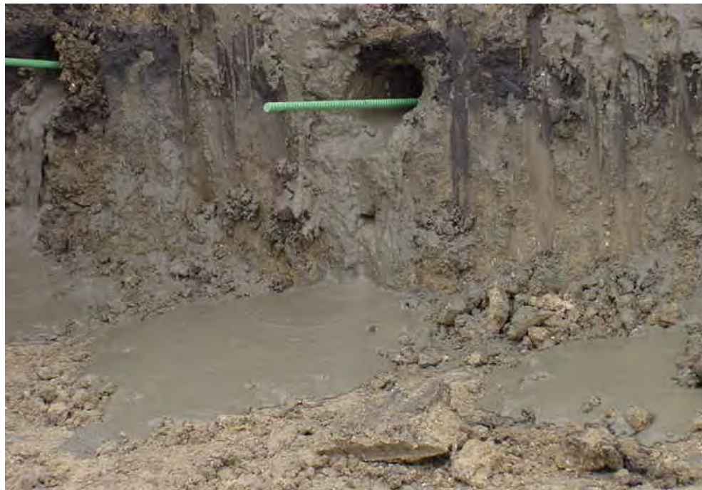
Figure 2.19 Excessively Fluid Mixes Cause Incomplete Grouting of Nail Head (Bird's Mouth Defects)
