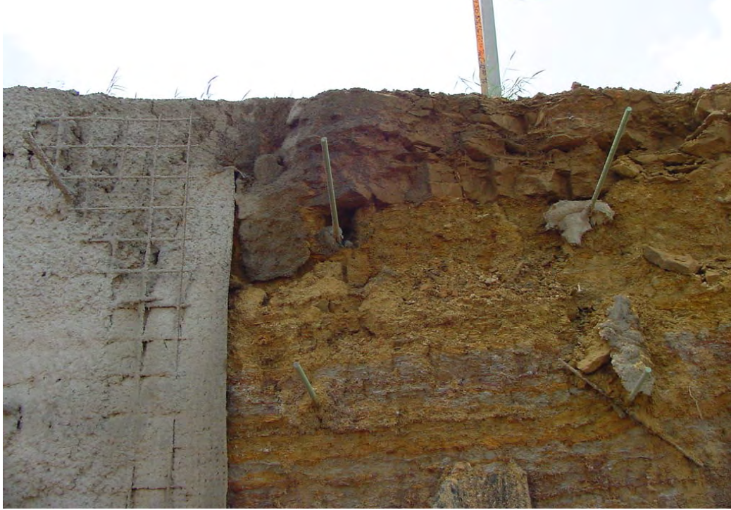
Figure 2.10 Long-Term Face Instability Caused by Drainage
