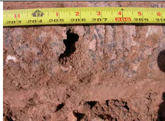
Minor defect at 17'2"
