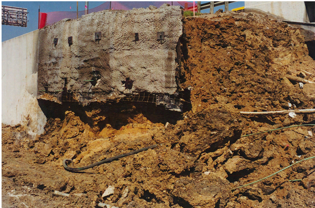
Figure 2.13 Failure of Wall Caused by Incomplete Grouting and Drainage
