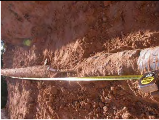
0~13'9" of the hole was fully grouted, and 13'9" ~15'9" of the hole was partially grouted, 15'9" to foam of the hole was fully grouted
