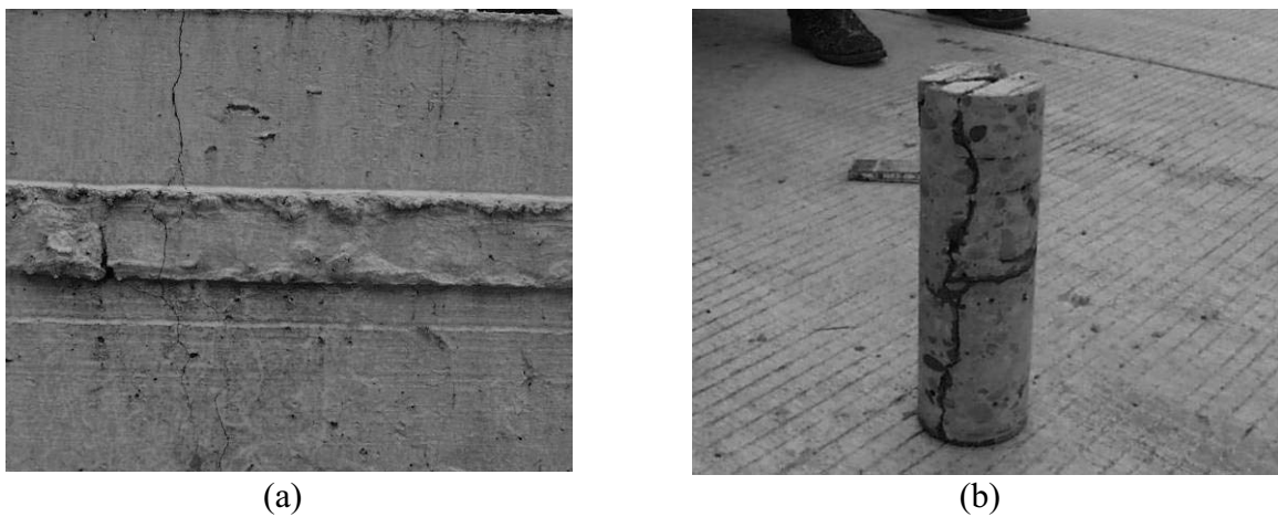
Figure 2.3: Horizontal cracking in new CRCP
