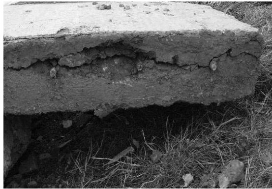
Figure 2.4: Horizontal cracking in CRCP
