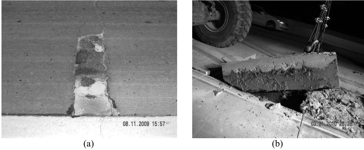
Figure 2.2: CRCP distress caused by horizontal cracking
