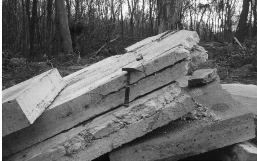
Figure 2.11: Slabs with horizontal cracks
