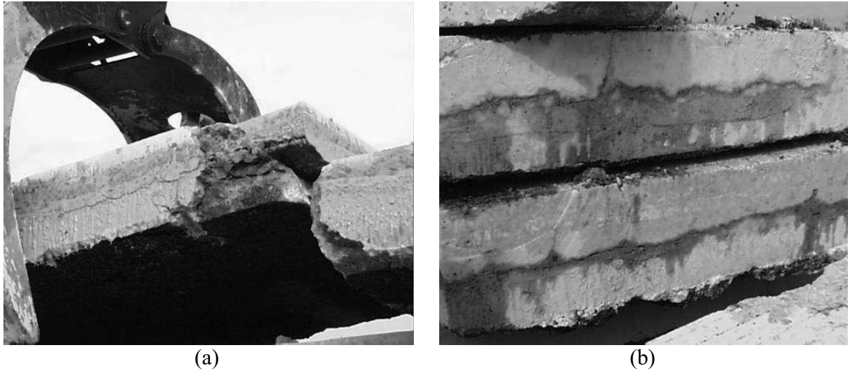
Figure 2.6: Horizontal cracks in slabs removed from IH30 in Paris District
