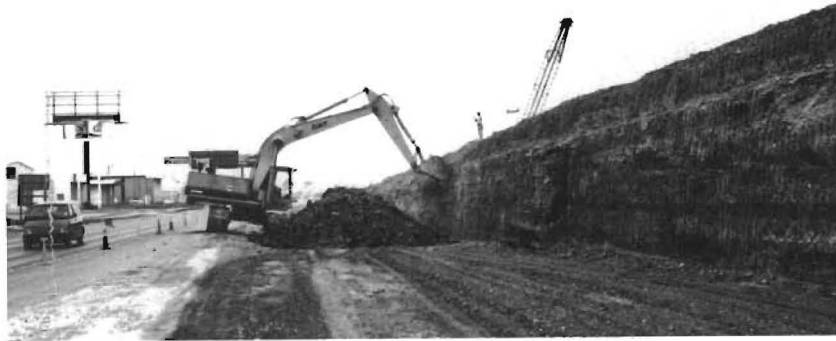
Fig. 3.1. Photograph of the procedure employed by the RSRW contractor in cutting back the constructed clay embankment to provide a vertical interface between the embankment and the to-be-constructed reinforced soil retaining wall and the cohesionless backfill.
