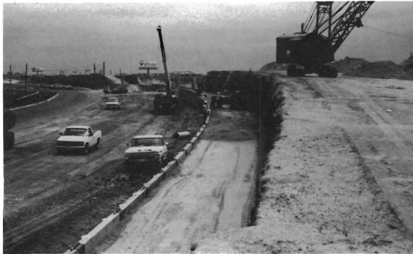
Fig. 3.2. Photograph of placement of the cohesionless backfill and the construction method employed by the contractor in constructing RSRWs on SH 358 overpasses.
