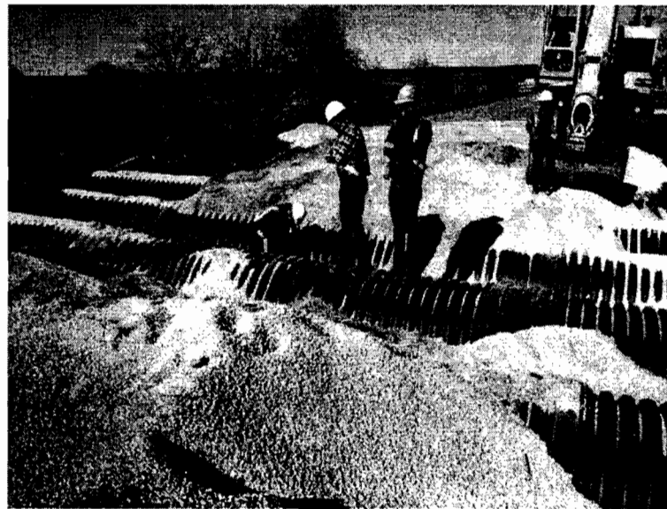
Figure 5.49 Wichita Falls Installation.
