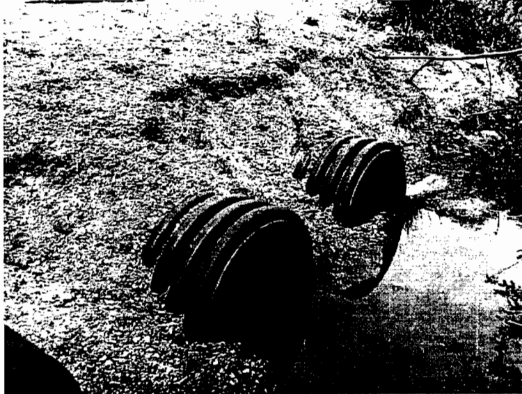
Figure 5.32 Erosion in Installation A1 in Atlanta District.
