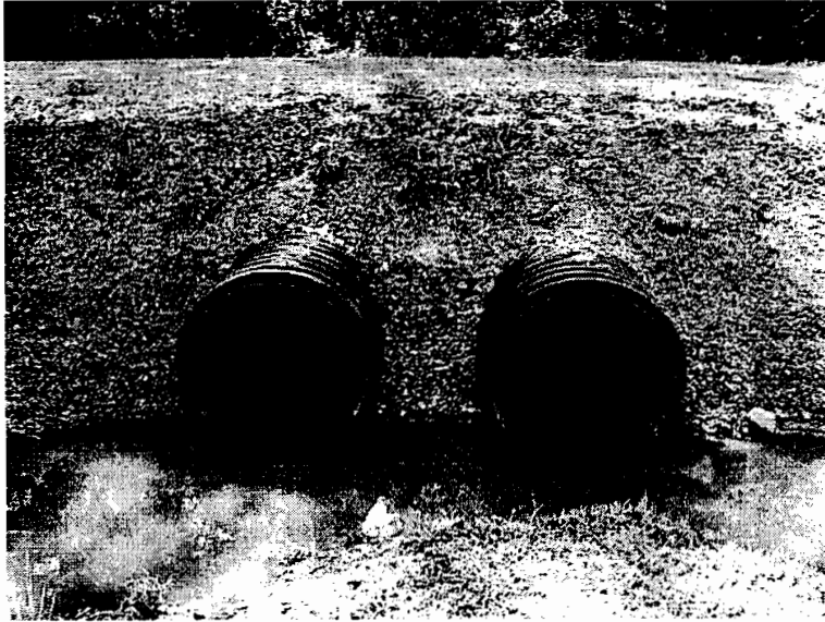
Figure 5.35 Installation A2 in Atlanta District.
