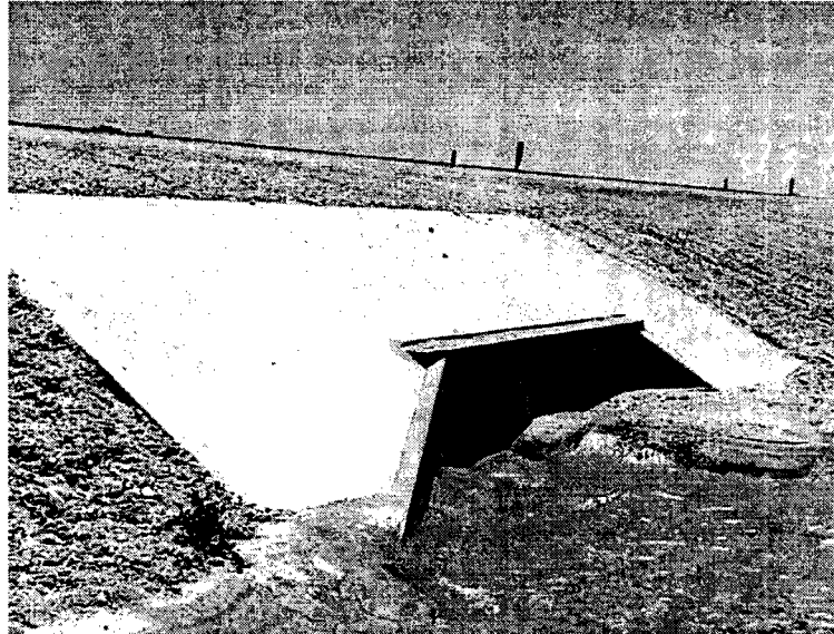
Figure 5.12 Silt Accumulation in Downstream End.
