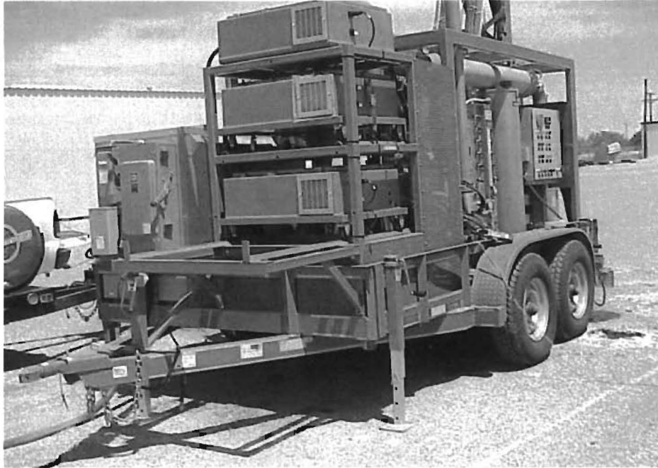
Figure 3 – Power Conditioning Unit (PCU)
