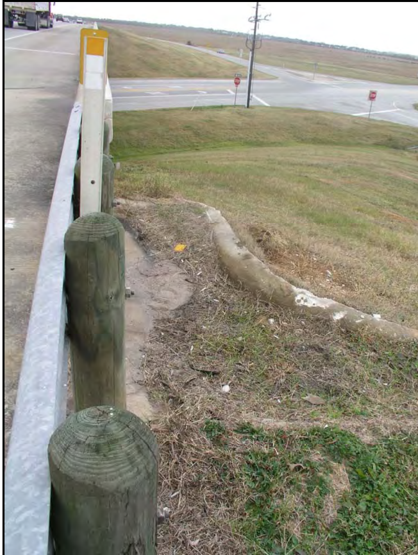
Figure 5.7 Effectiveness of Drainage Flume Impaired by Weeds and Debris Collection
