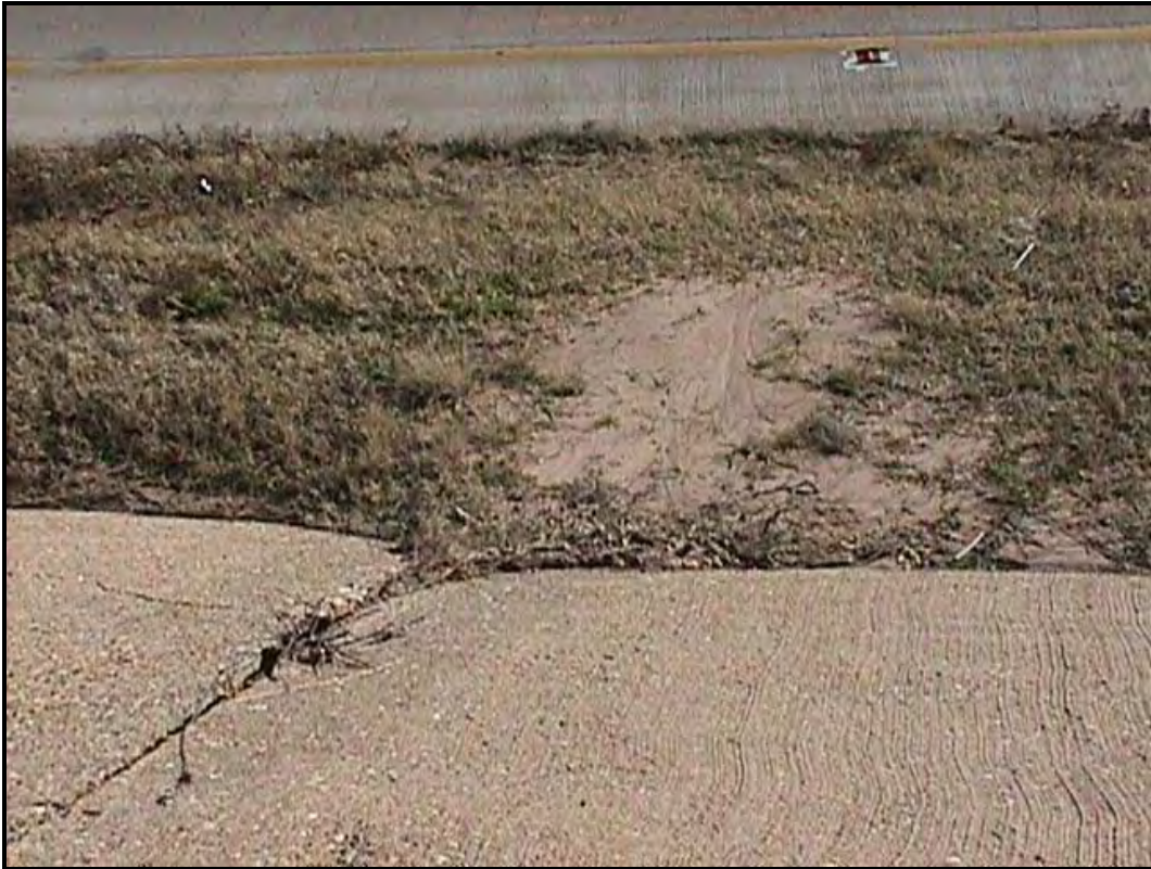
Figure 5.2 Signs of Embankment Fill Erosion at IH-27 Overpass over 4 th Street in Lubbock District
