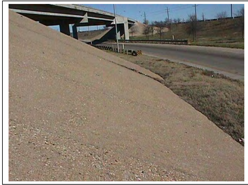
Figure 4.4 Differential Settlement of Riprap Slab (Side View)
