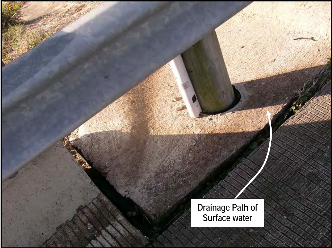
Figure 5.11 Open Joint between Approach Slab and Mow Strip
