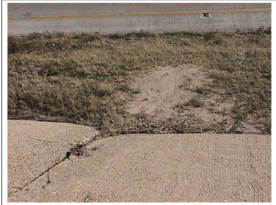
Figure 4.2 Top View of Riprap with Washed-Out Fines at Toe
