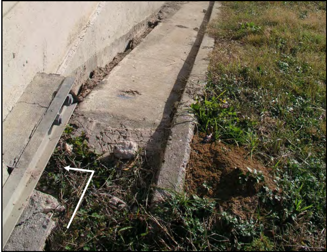
Figure 5.6 Badly Damaged Drainage Flume Allowing Water to Flow Underneath Approach Slab
