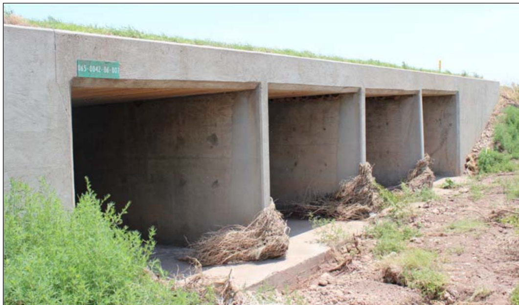
Figure 1.1 Structure 25-065-0042-06-007, upstream end, a 4-span, 9'x7' reinforced concrete box culvert, constructed 1934, widened 1978, Donley County, Childress District
