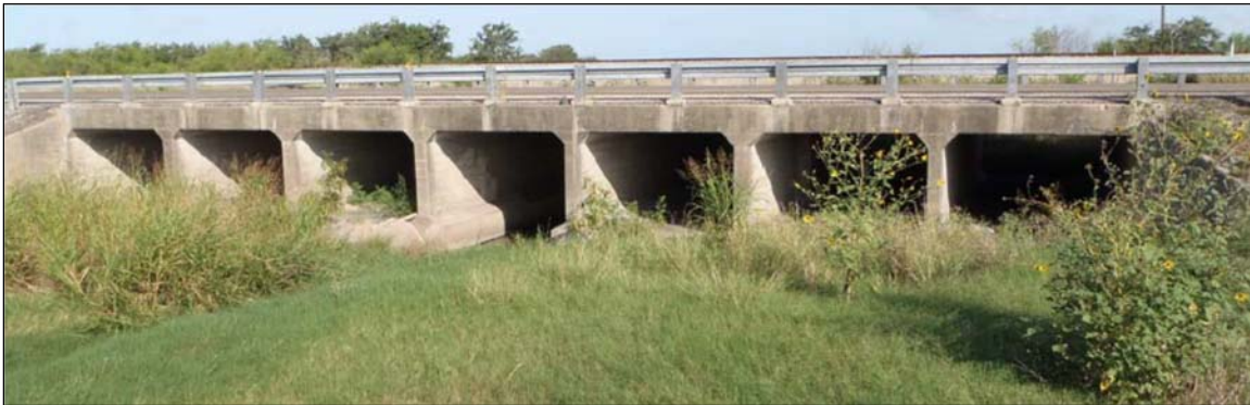
FIG 1. Complex 7-span reinforced concrete box culvert; Nueces County, Corpus Christi District; original construction 1924, widened/ lengthened 1947; Structure #161780010202005.
