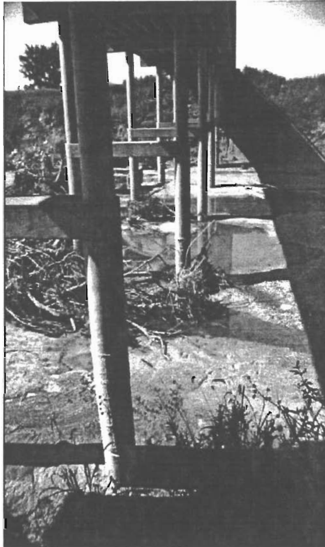
Figure 20. Photograph of view north to show the channel cross section at the bridge. The level of the channel at the time the piers were poured can be seen on by the markings on the two closest piers. Erosion of the channel bed is endangering all the bridge support structures and both abutments.
