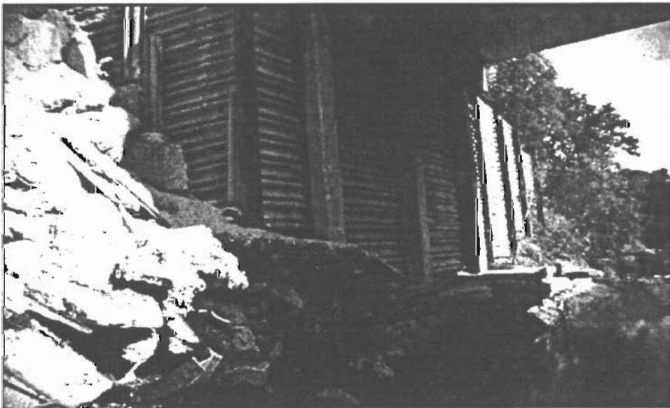
Figure 10. Concrete rubble dumped on the upstream upside of the abutment was covered in-place with poured concrete in an attempt to slow erosional retreat of the bank. Such “unconventional” measures pose an aesthetic and perhaps an environmental concern.
