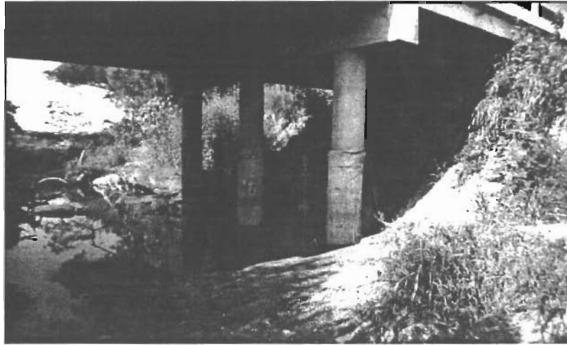
Figure 13. Erosion of the channel bed is endangering bridge support structures and abutments, also resulting in environmental and aesthetic problems. Artificial straightening in the trunk stream channel downstream (Sulfur River) caused at least a 2-meter drop in channel bed elevation in this tributary drainage.
