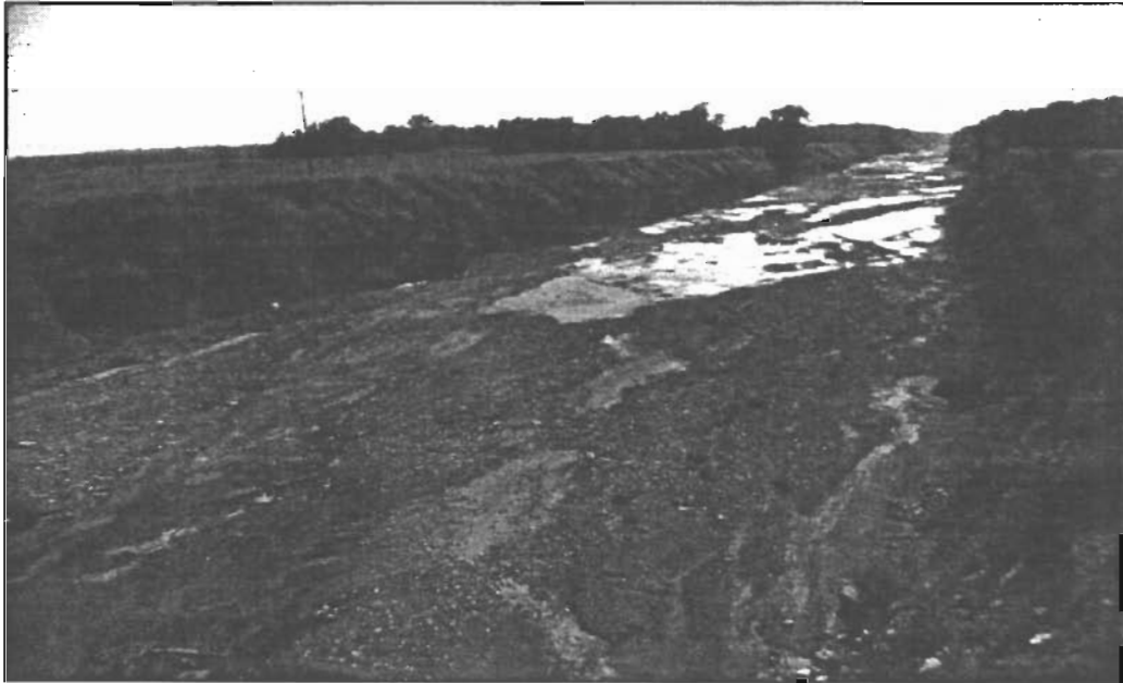
Figure 21. Photograph with a view east to show a view of the channel downstream from the bridge. Natural channel alluvium has been scoured away by erosion. The banks are subject to slope failure and to erosion. The channel bottom is bedrock with a few scattered gravel drifts over the surface.
